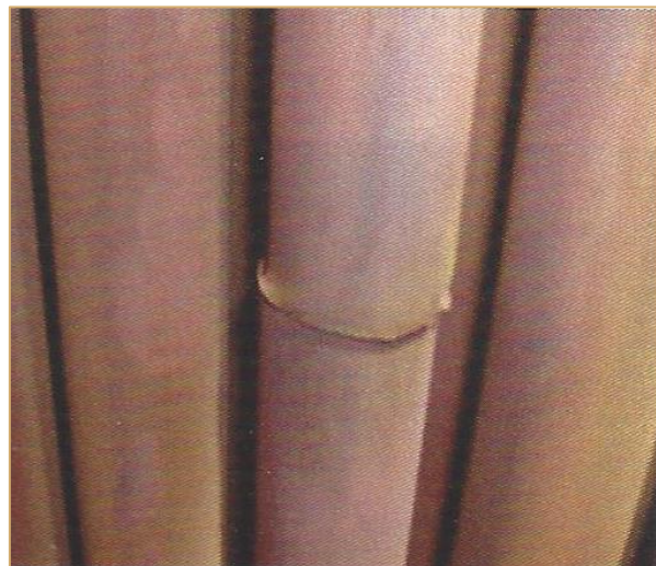
Figure 6-1 Condenser tube broken by mechanical fatigue [Hutin, 2016].
