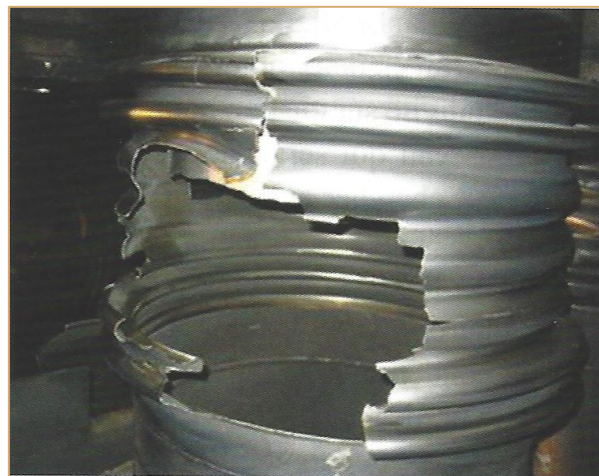
Figure 6-3 Steam extraction expansion joint, corrugated steel severely torn out [Hutin, 2016].
