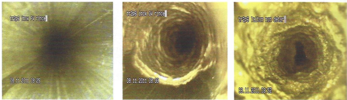
Figure 6-2 View of condenser tubes ID. Left: clean tube. Middle: tube with scale deposits. Right: tube almost plugged by deposits [Hutin, 2016].
